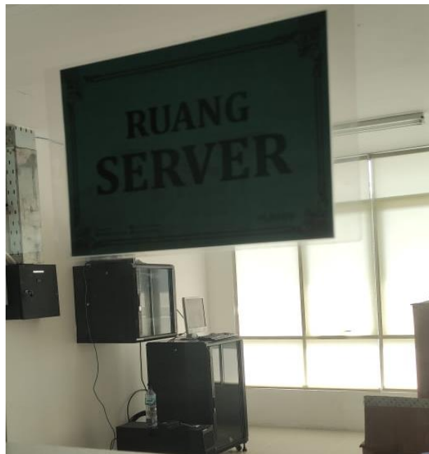
Gambar: Ruang Server
